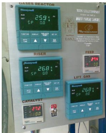
Figura 4.10. Panel de control
