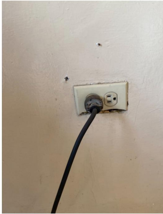
Figure 13. Status of Electrical Outlets
