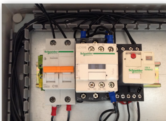
Fig 71. Braker, contactor y relay
